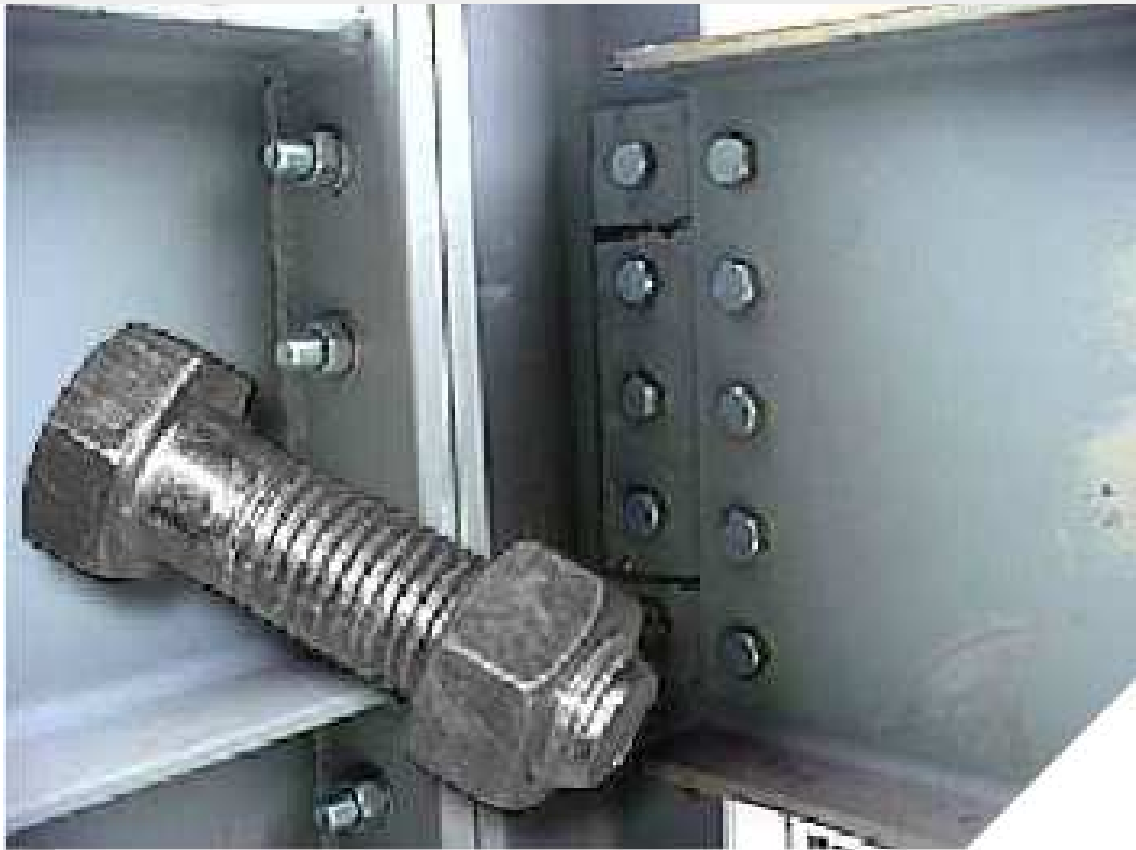
Bolts and fixings
